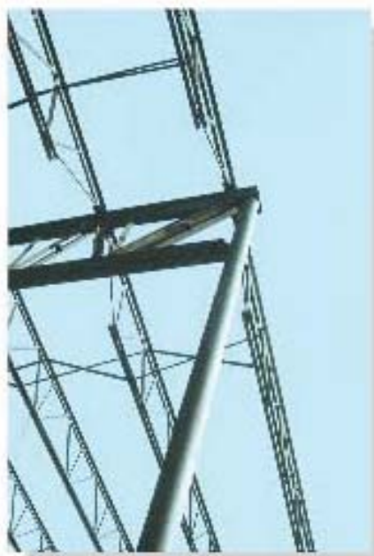
Typical example of a column used to support an eccentric roof loading.
