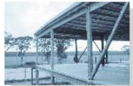
Steel rapidly loses its strength when heated. For this reason engineers often require main structural members to be insulated in case of fire.
