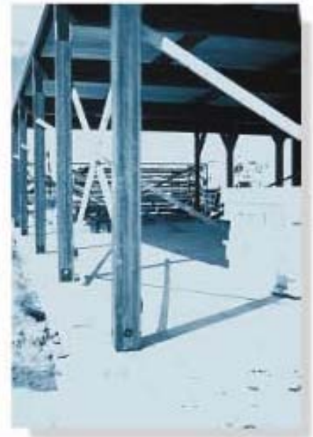
These timber columns can be considered pinned at their bottom and fixed connected to the beams at their tops.
