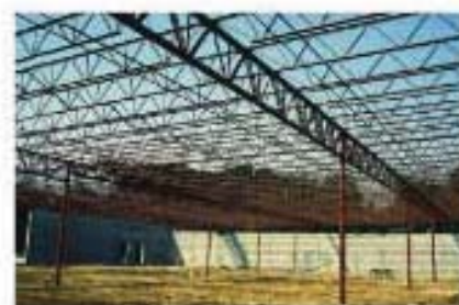
Typical interior steel pipe columns used to support the roof of a single-story building.
