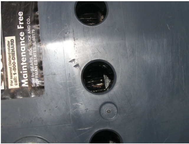
FIGURE 51-1 A visual inspection on this battery shows the electrolyte level was below the plates in all cells.
