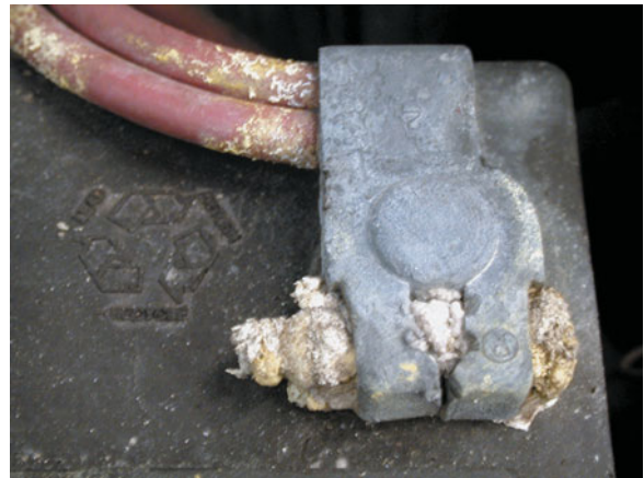
FIGURE 51-2 Corrosion on a battery cable could be an indication that the battery itself is either being overcharged or is sulfated, creating a lot of gassing of the electrolyte.
