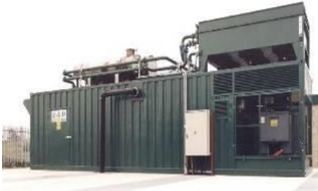
1MW generator at Buckden - Biogas Association
