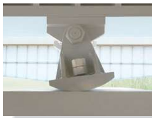
The rocker support for this bridge girder allows horizontal movement so the bridge is free to expand and contract due to a change in temperature. (4)
