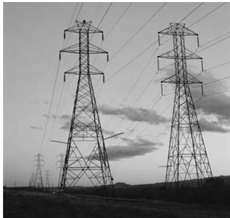
FIGURE 4.26 Electrical power transmission tower and line.
